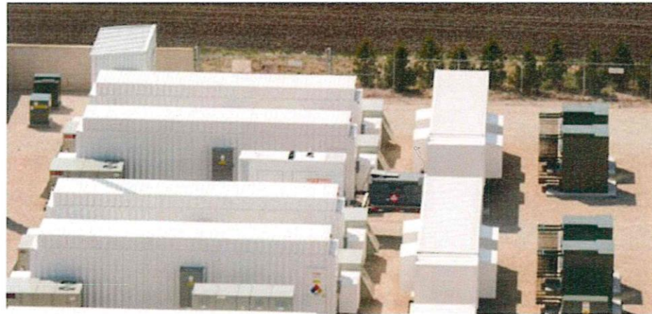
Battery containers – typical view
