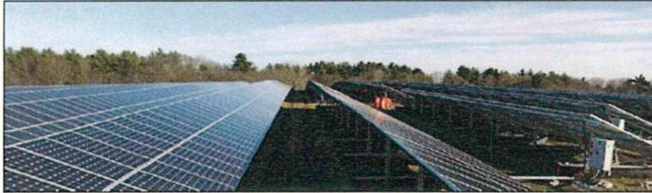
Solar Panels – typical view
