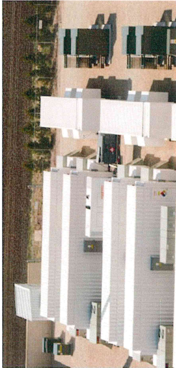
Battery containers – Typical view
