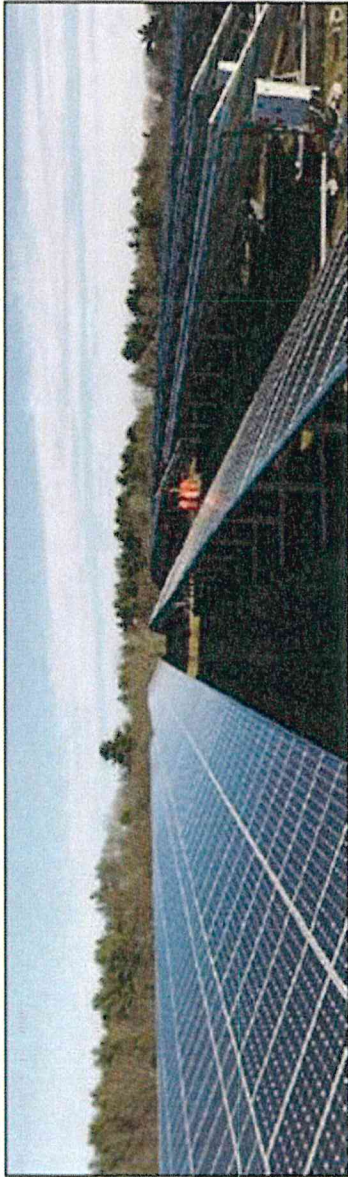
Solar Panels – Typical view
