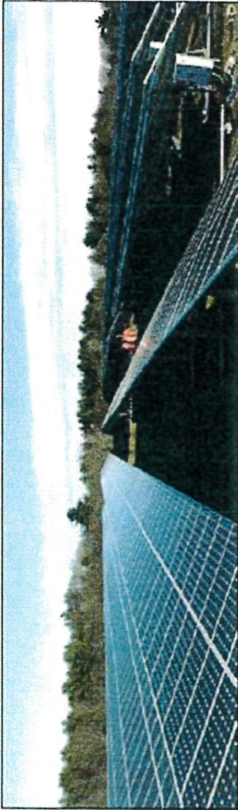
Solar Panels – Typical view
