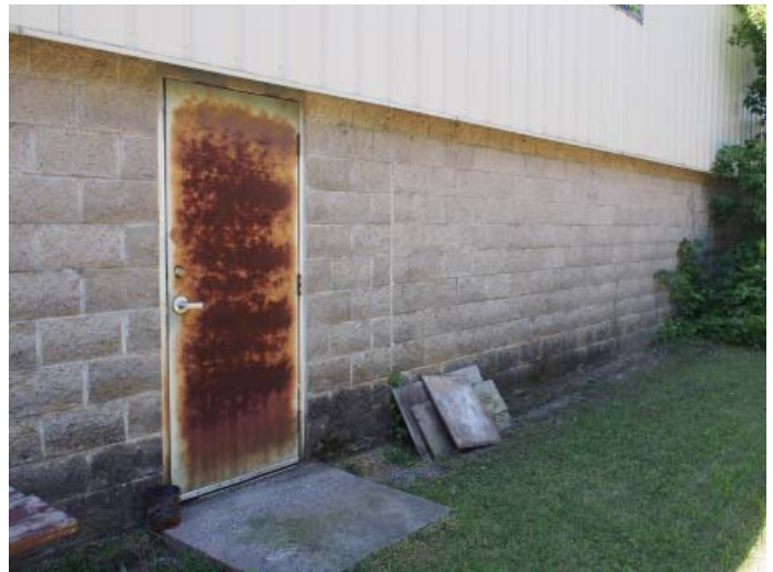
Figure B.I.9: Hollow metal door and frame rusting and signs of moisture damage at masonry wall along grade
