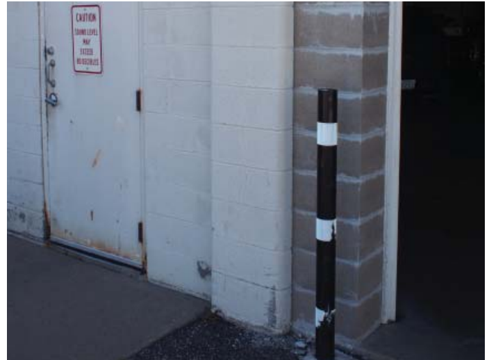
Figure B.3.2: Exterior masonry jambs have been repaired at overhead door but lack proper sealing/finishing
