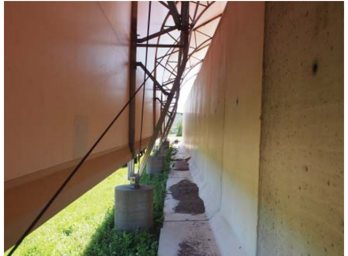
Figure B.4.2: Precast wall panels and concrete foundation piers along exterior wall are in good condition
