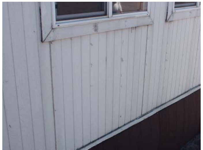
Figure B.5.4: Exterior cladding is showing age and needs to be painted
