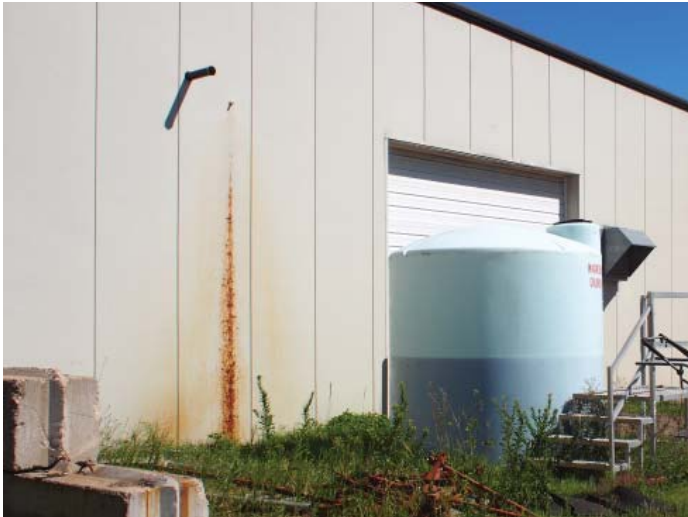
Figure B.2.5: Condensate drain is located high on the wall causing rust stains on South facade
