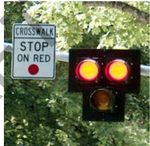
Proposed PHB or HAWK System Light until Bunker Lake Blvd/Center Street intersection is signalized
