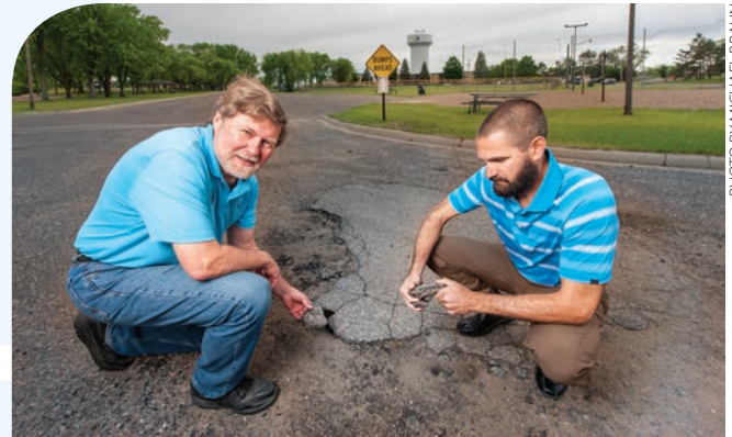
Mayor Dietz and City Engineer Femrite look at distressed pavement in need of reconstruction.
