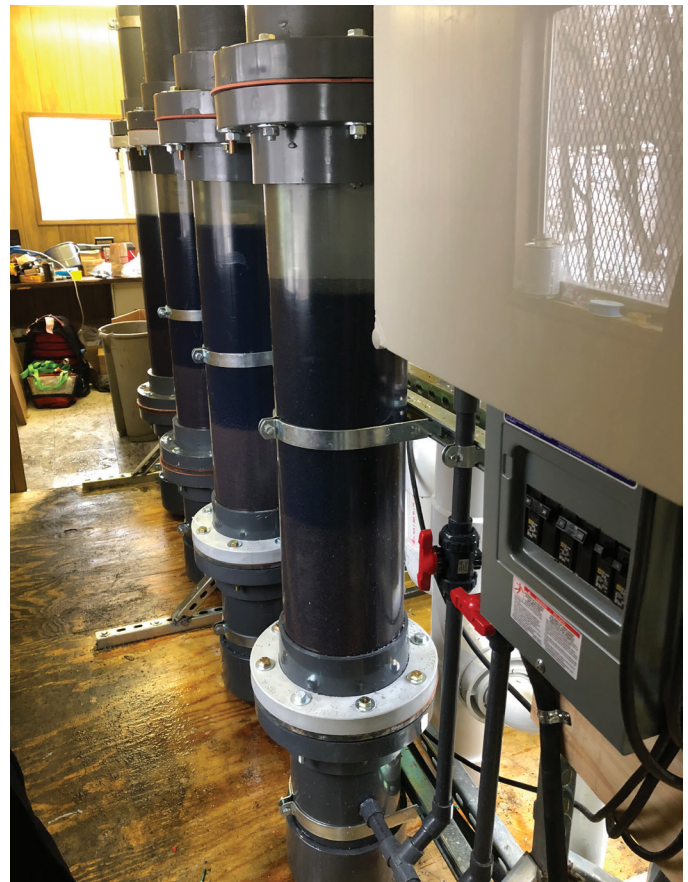
SEH Pilot Filters – Biological Ammonia Removal
