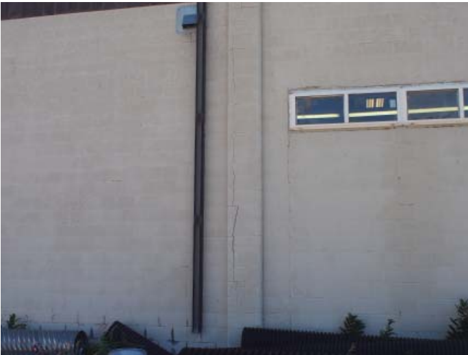
Figure B.3.6: Vertical cracks are visible in masonry pilaster at West facade
