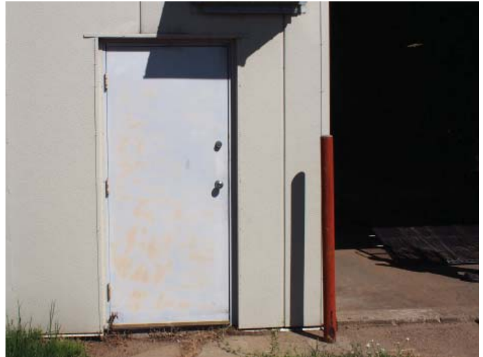
Figure B.2.2: Hollow metal door and frame on South facade is rusting
