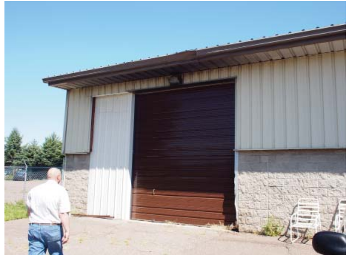
Figure B.1.2: No code-required exit door
