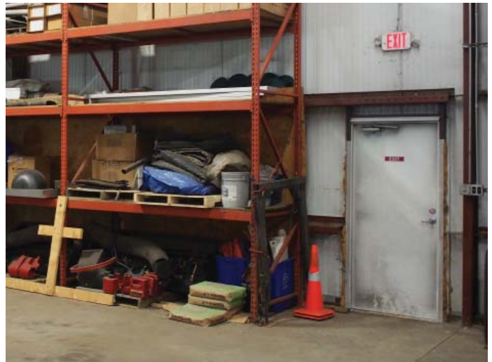
Figure B.2.3: Northwest exit door is stuck in closed position, does not meet code
