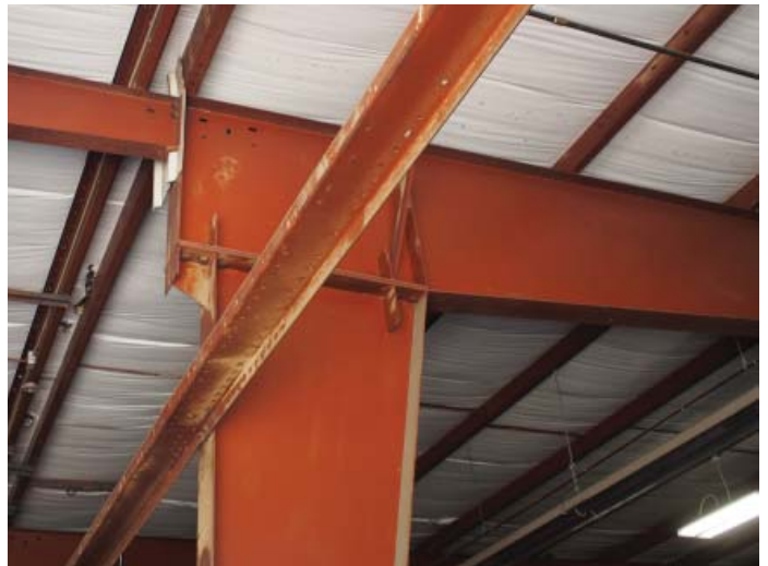
Figure B.2.8: Steel structure is showing evidence a failing finish and rusting
