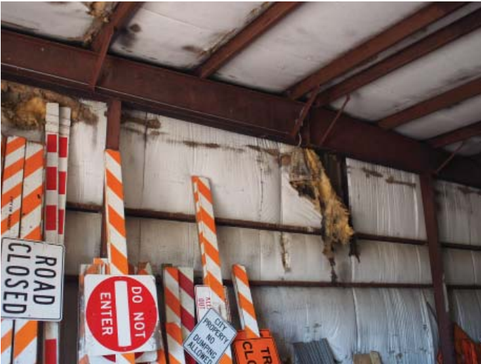
Figure B.I.5: Damaged / torn insulation and vapor barrier
