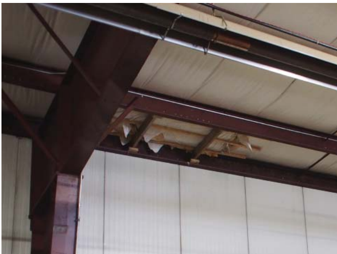
Figure B.2.6: Insulation and vapor barrier is damaged
