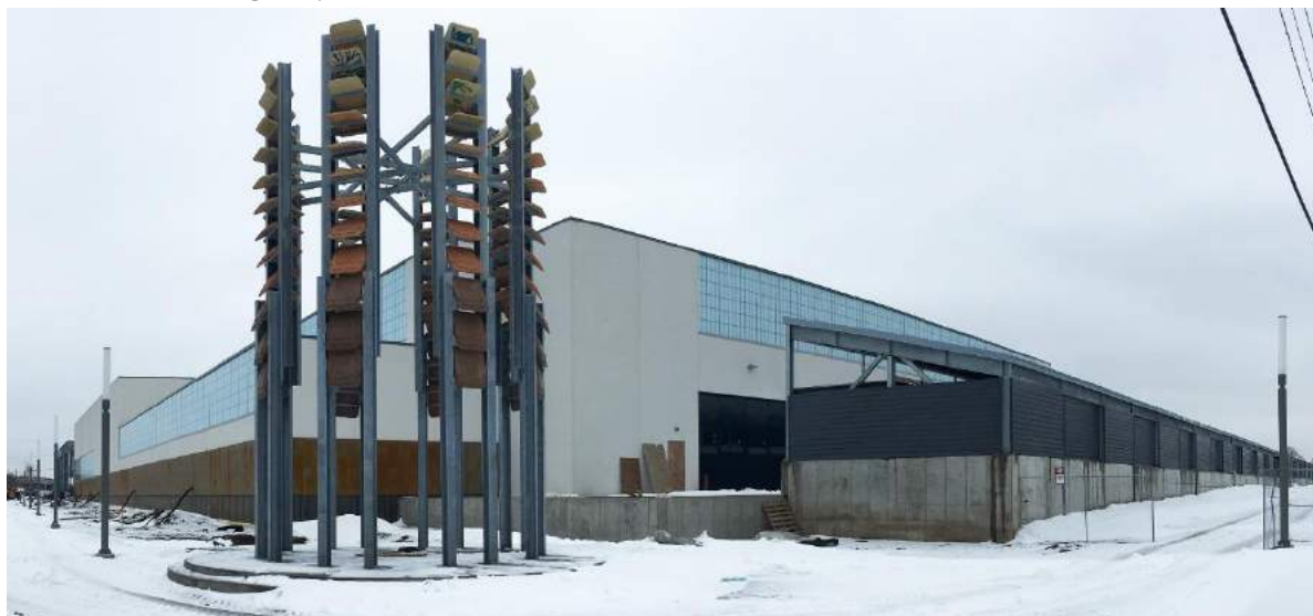
Construction - Covered Cold Storage (right), Warm Vehicle Storage (background), Public Art Installation (foreground)
