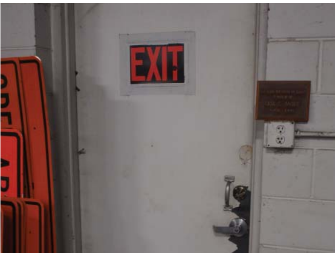
Figure B.1.12: Exit door has deadbolt with thumb-turn which is not allowed by code
