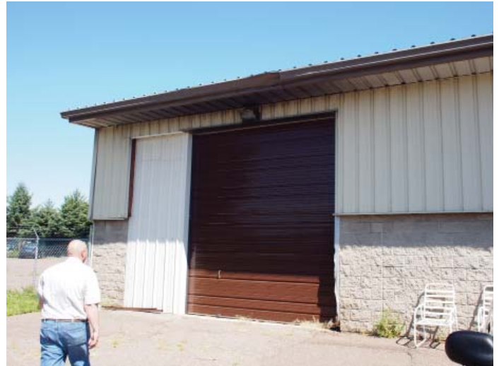
Figure B.1.2: No code-required exit door
