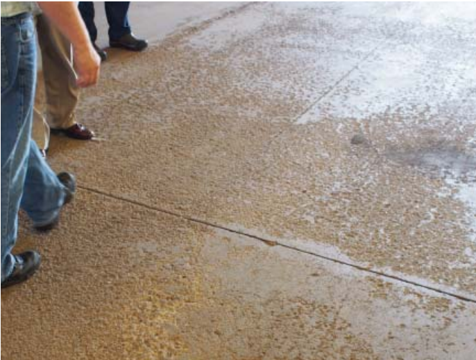
Figure B.3.11: Concrete slab on grade is heavily worn, spalling and cracking
