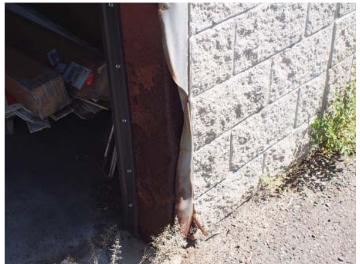
Figure B.1.4: Overhead door jamb damaged and rusting
