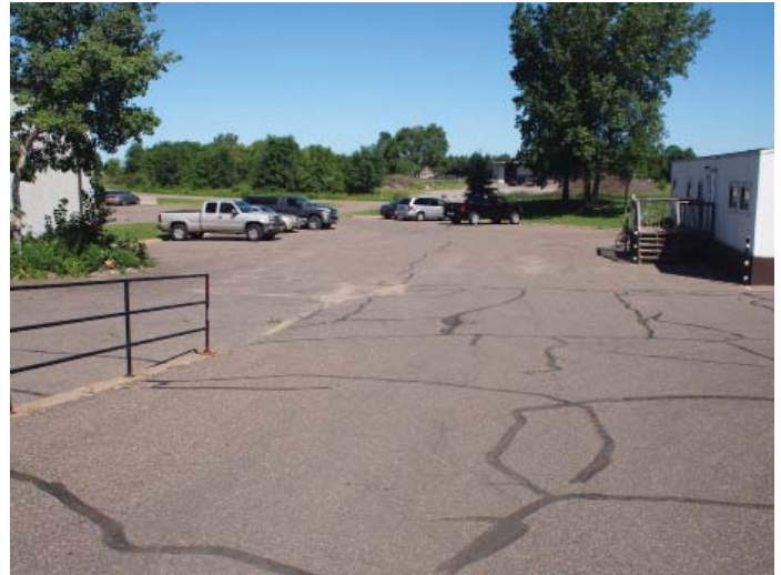
Figure B.6.3: On-site pavement has multiple cracks and has less than 10 years of useful service life remaining
