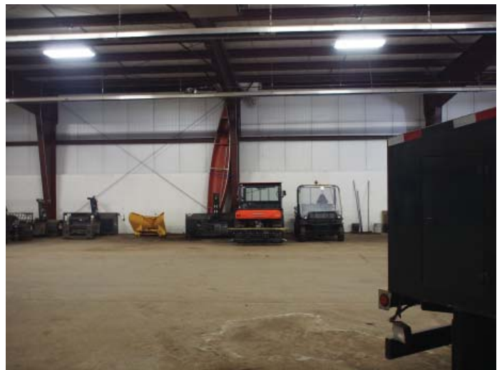
Figure B.2.4: Building lacks floor drains in main storage area creating slip hazards from wet vehicles
