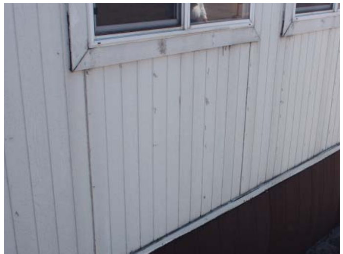
Figure B.5.4: Exterior cladding is showing age and needs to be painted
