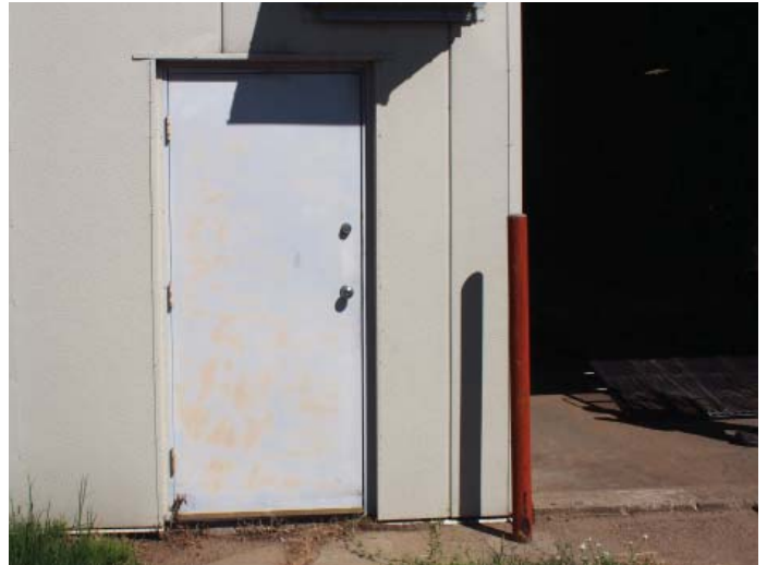
Figure B.2.2: Hollow metal door and frame on South facade is rusting
