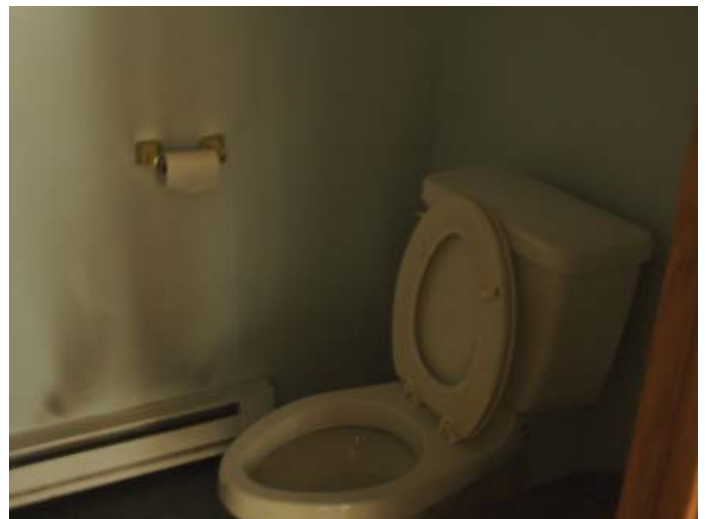
Figure B.1.15: Restroom is not handicap accessible
