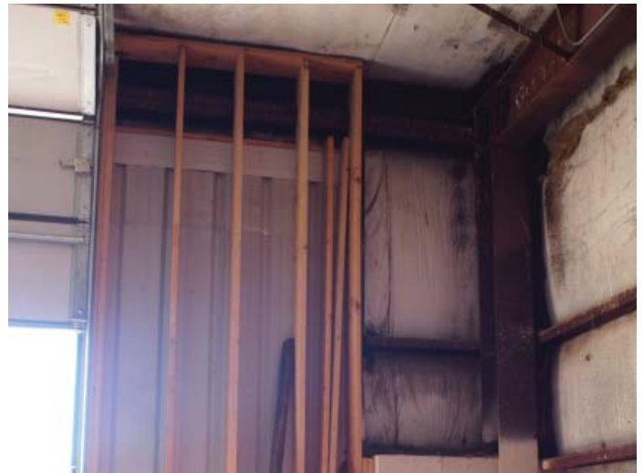
Figure B.1.3: Overhead door opening infilled with metal panel and wood studs
