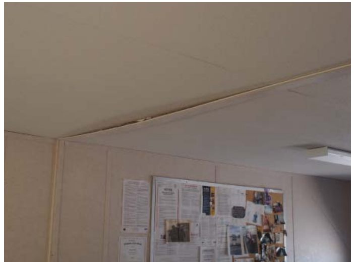
Figure B.5.3: Ceiling is starting to sag and separate at seam of trailer
