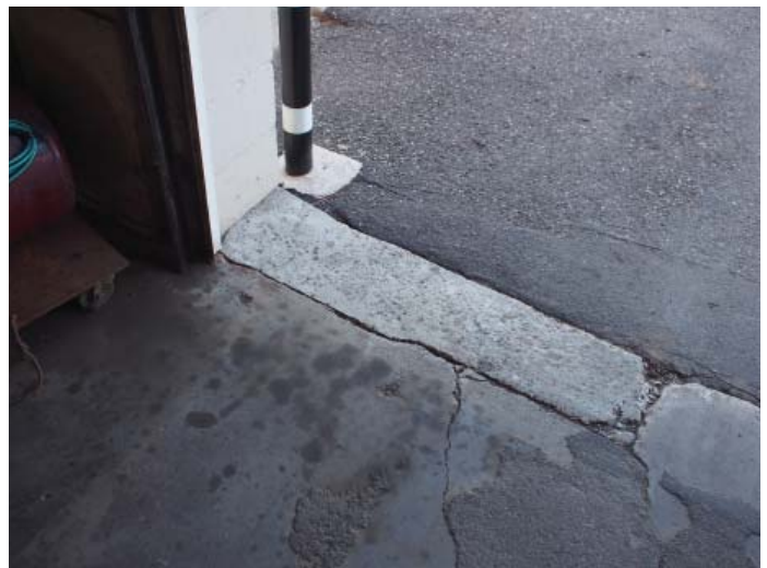
Figure B.3.4: Concrete apron at overhead doors is cracking and spalled
