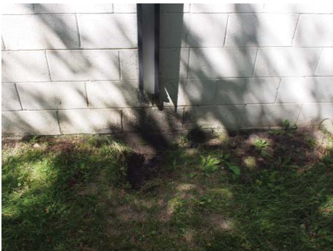
Figure B.3.7: Downspouts have eroded soil at base of wall/foundation causing potential drainage issues
