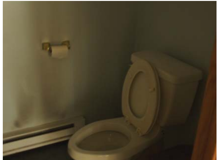
Figure B.1.15: Restroom is not handicap accessible
