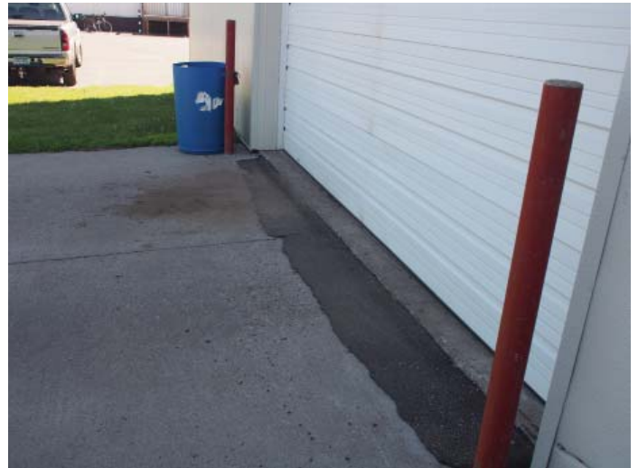
Figure B.2.9: Settling of concrete apron at North overhead door has necessitated asphalt patching
