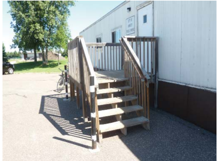
Figure B.5.2: Main entrance lacks signage directing to accessible entrance
