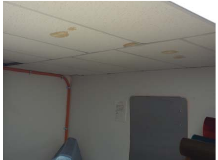
Figure B.1.14: Evidence of roof leaks in sign shop area
