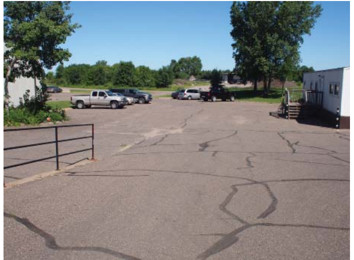
Figure B.6.3: On-site pavement has multiple cracks and has less than 10 years of useful service life remaining
