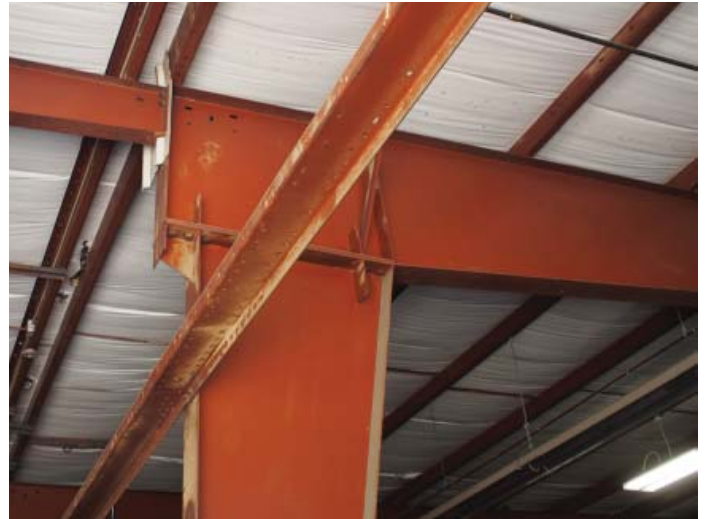
Figure B.2.8: Steel structure is showing evidence a failing finish and rusting
