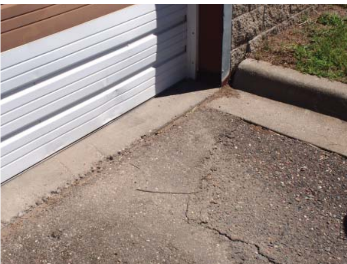
Figure B.I.7: Depressed asphalt at door threshold causing ponding and drainage issues
