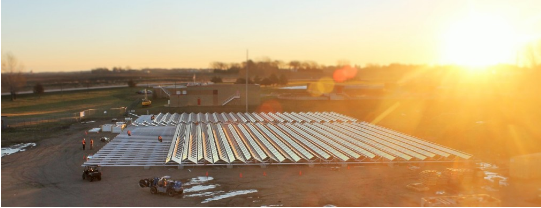
Workers install the last panels as the sun rises over the City of Hutchinson's new solar PV project, the largest on a landfill in Minnesota, and the first ballast-mounted on a brownfield. ( https://www.ci.hutchinson.mn.us/december-2-grand-opening-ceremony-landfill-mounted-solar-pv-system/ )
