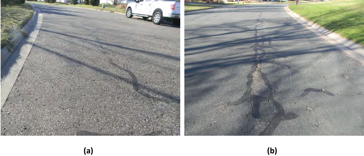
Figure 14. Possible contribution of chip seal to advanced cracking in (a) unsealed and (b) chip-sealed pavement on Blue Heron Road in Woodbury, MN
