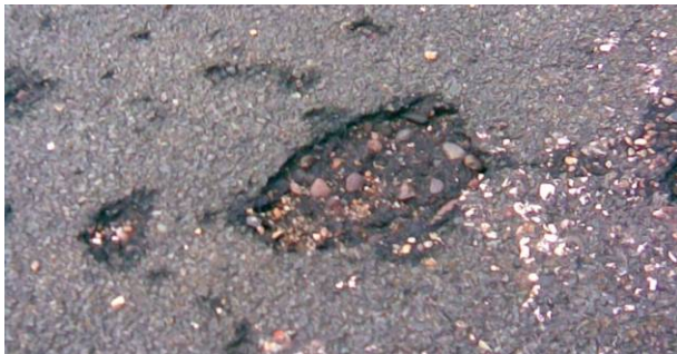
Figure 1.1. Early stage of HMA deterioration under a chip seal (251 Reid).
