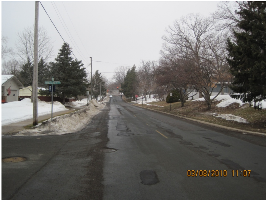
Figure 2: Asphalt deterioration under chip seal.
