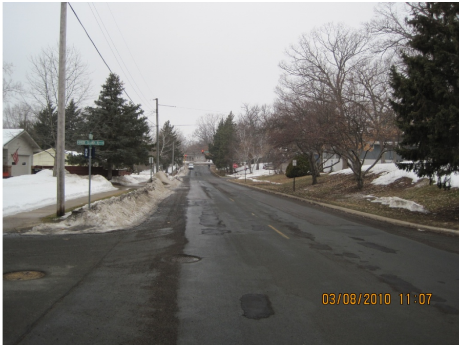
Figure 2: Asphalt deterioration under chip seal.
