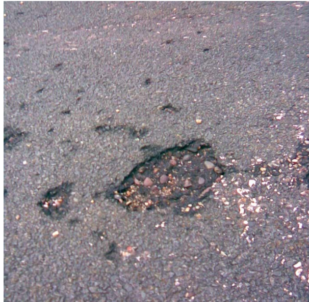
Figure 1. Early stage of HMA deterioration under a chip seal (251 Reid).
