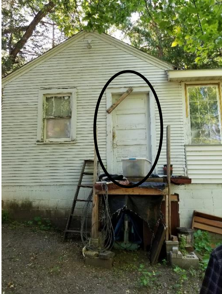
Exhibit 1: Back door with safety issue
