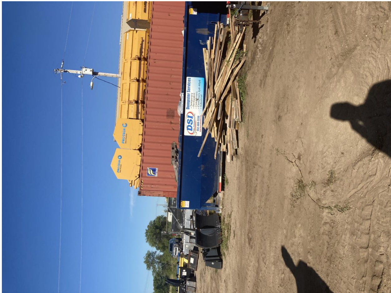
Outdoor storage of construction materials (violation of chapter 30)
