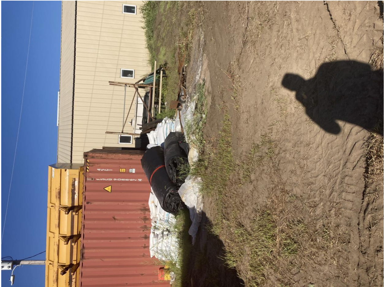
Continued – construction materials in piles (violation of chapter 30)
