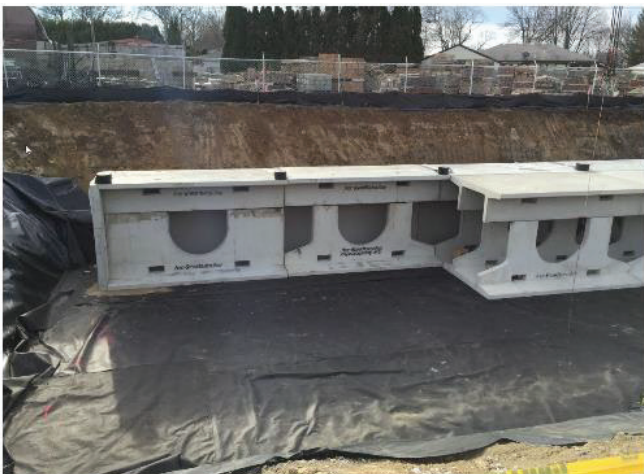
Exhibit 2: Example concrete vault storage tank (Storm Trap).
