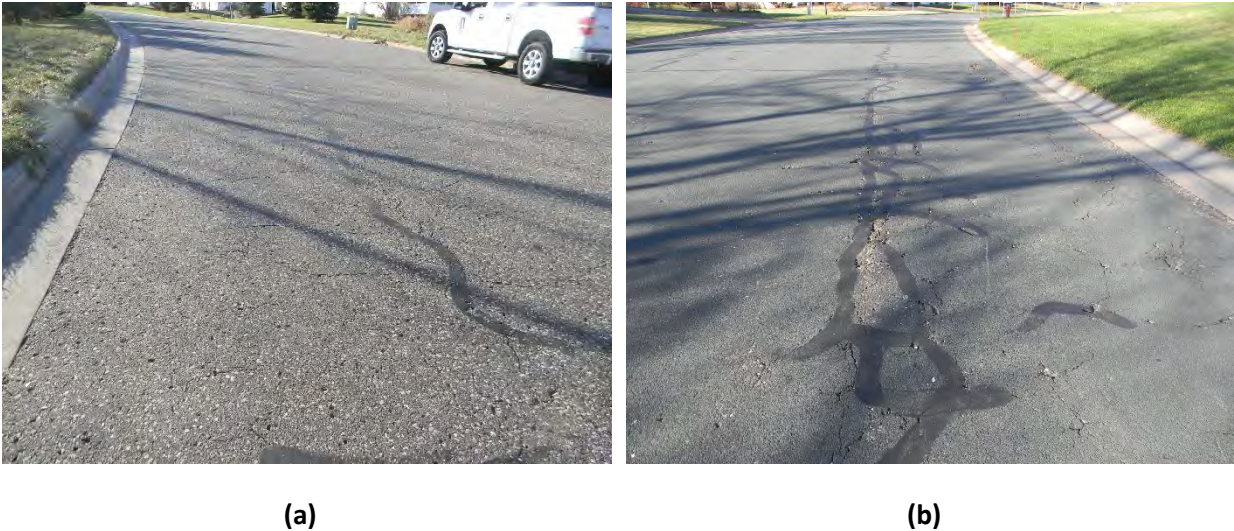
Figure 14. Possible contribution of chip seal to advanced cracking in (a) unsealed and (b) chip-sealed pavement on Blue Heron Road in Woodbury, MN
