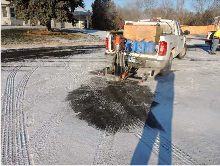
Figure I-7. Coring operations and sample core extracted from Heritage Circle in Burnsville, MN
