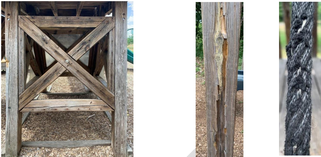
Figures 21-23: (from left to right) Splintered wood on horizontal and diagonal supports; Splintered wood on support for swing set; Worn rope covering on climbing wall
