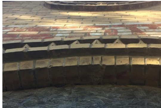
Figure 6 – Red Paint on Overhead Framing
