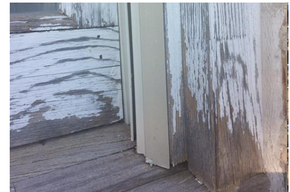
Figure 27 – Paint Chipping on Window Frame
