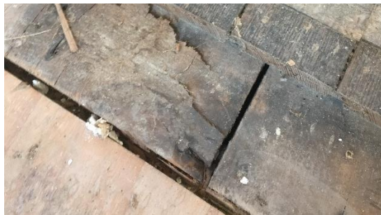
Figure 35 – Bathroom Water Damage
