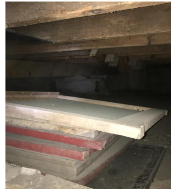
Figure 51 – Crawl Space with Debris
