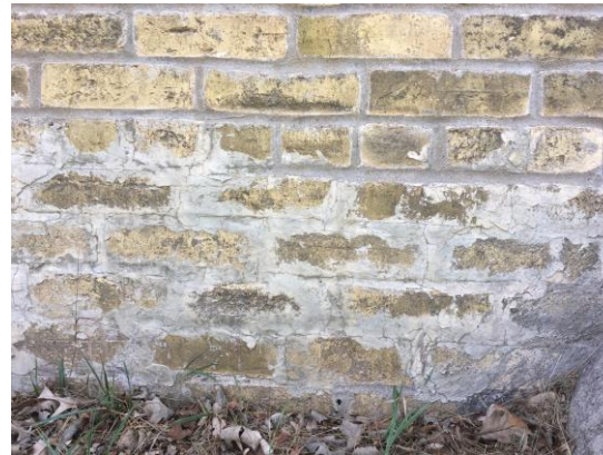
Figure 23 – Deteriorated Brick with Mortar
