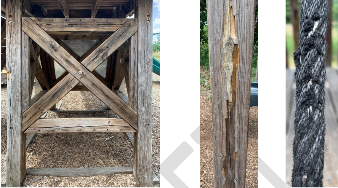
Figures 3-5: (from left to right) Splintered wood on horizontal and diagonal supports; Splintered wood on support for swing set; Worn rope on climbing wall
