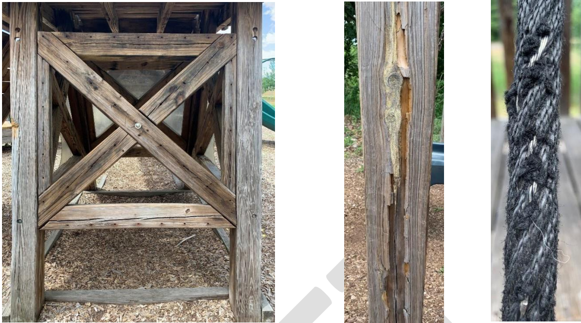
Figures 21-23: (from left to right) Splintered wood on horizontal and diagonal supports; Splintered wood on support for swing set; Worn rope on climbing wall
