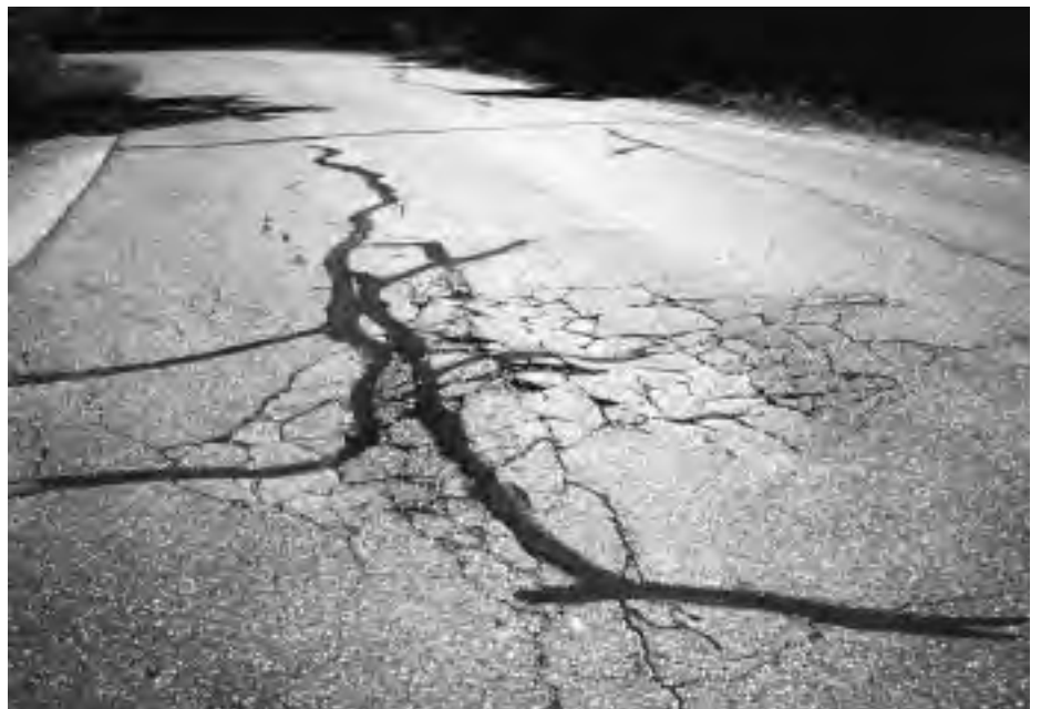
► Frost heave damage from spring break-up.
