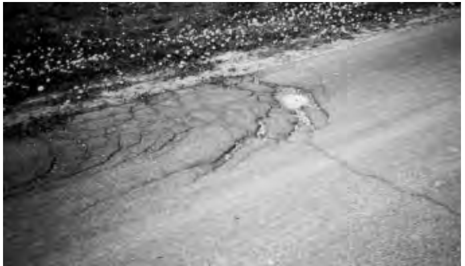
► Crescent-shaped cracks characteristic of slippage.
