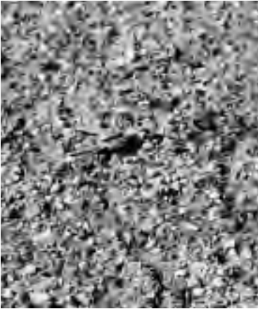
Severe raveling with ▼ extreme loss of aggregate.
