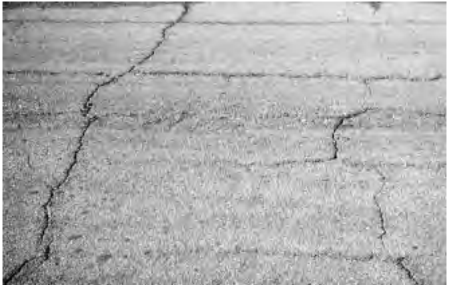
▶ Intermediate-size block cracking, 1'-5' across with open cracks.
