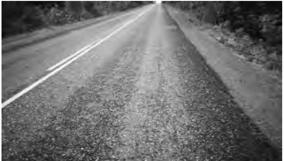
► Moderate to severe raveling in wheel paths.
