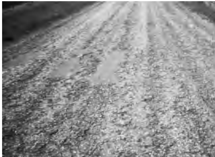
◀ Severe raveling and loss of surface material.
