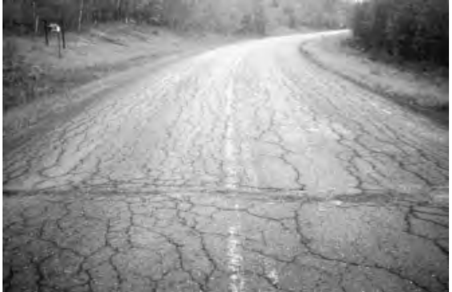
► Extensive alligator cracking. Pulverize and rebuild.
