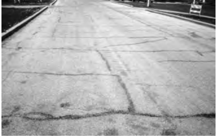
▶ Large blocks, approximately 10' across.
