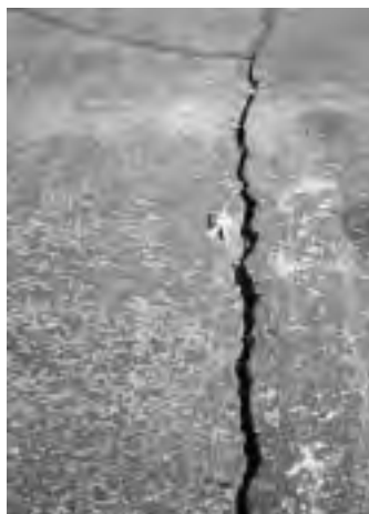
▲ Open crack – 1/2" or more in width.
