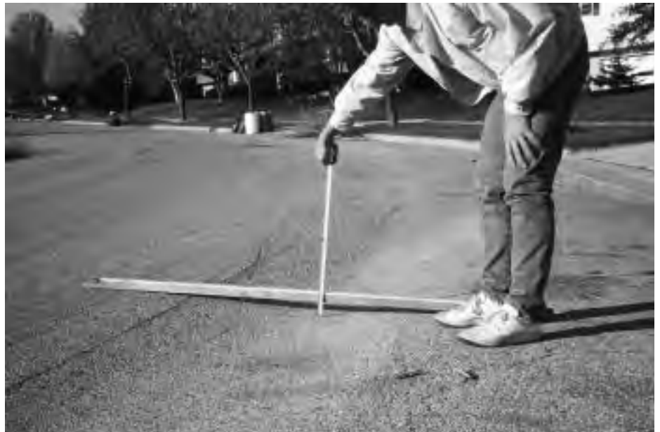
► Severe settling from utility trench.
