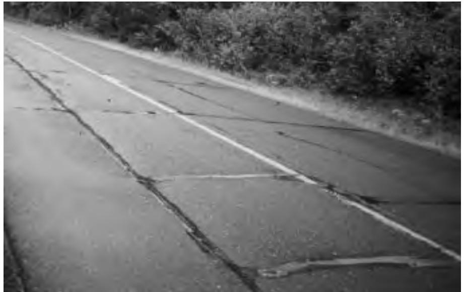
► Concrete joints reflected through bituminous overlay.
