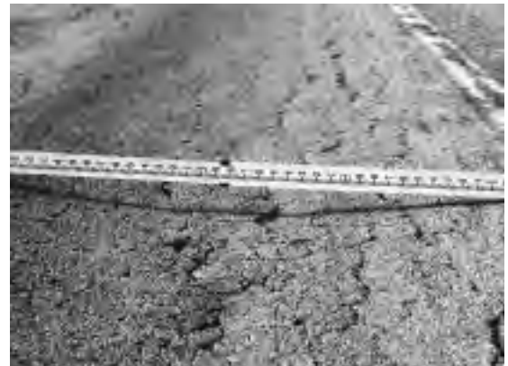
▲ Severe rutting. Strengthen base and reconstruct.
