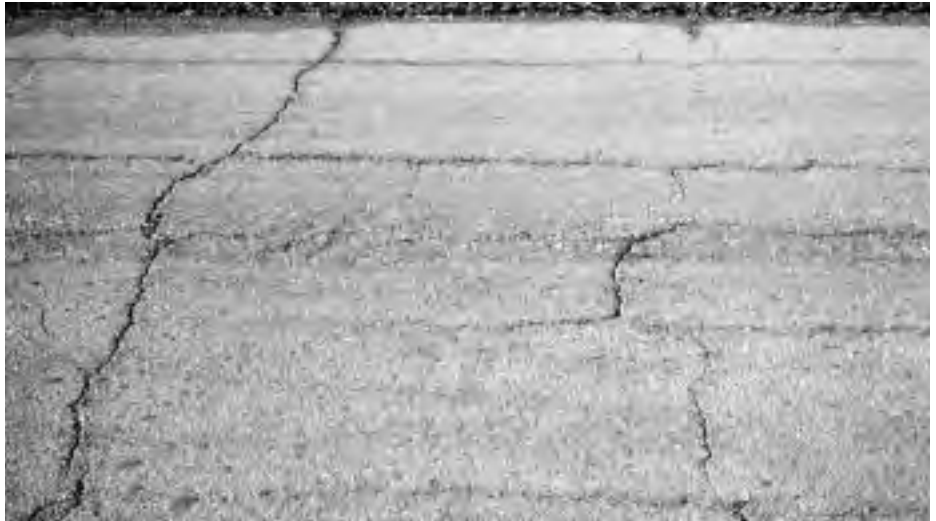
▼ Block cracking with open cracks.
