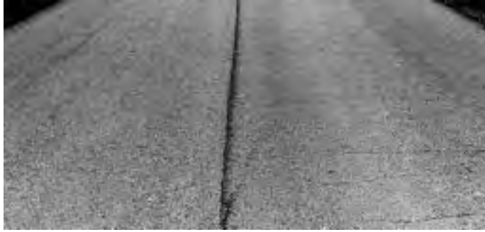
Centerline crack (still tight). ▶
