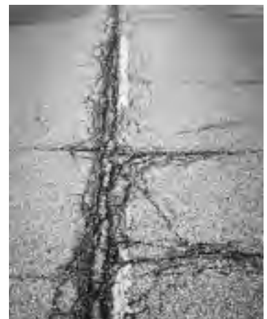
▲ Pavement ravels and erodes along open cracks causing deterioration.
