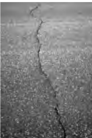
▲ Tight cracks less than 1/4" in width.
