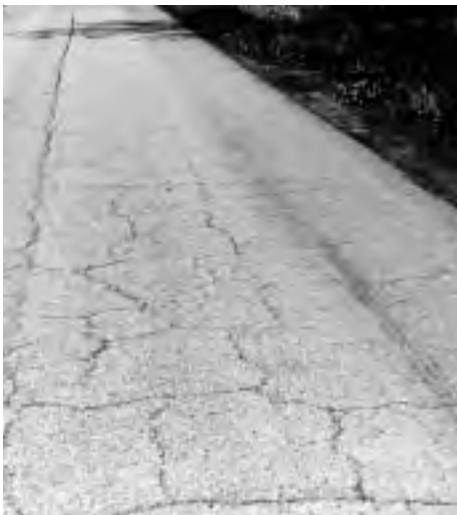
▲ Extensive block cracking in an irregular pattern.
