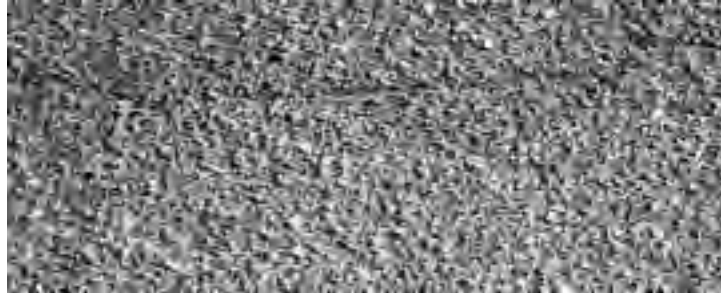
◀ Slight raveling. Small aggregate particles have worn away exposing tops of large aggregate.
