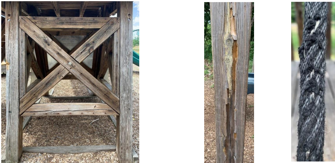
Figures 21-23: (from left to right) Splintered wood on horizontal and diagonal supports; Splintered wood on support for swing set; Worn rope covering on climbing wall
