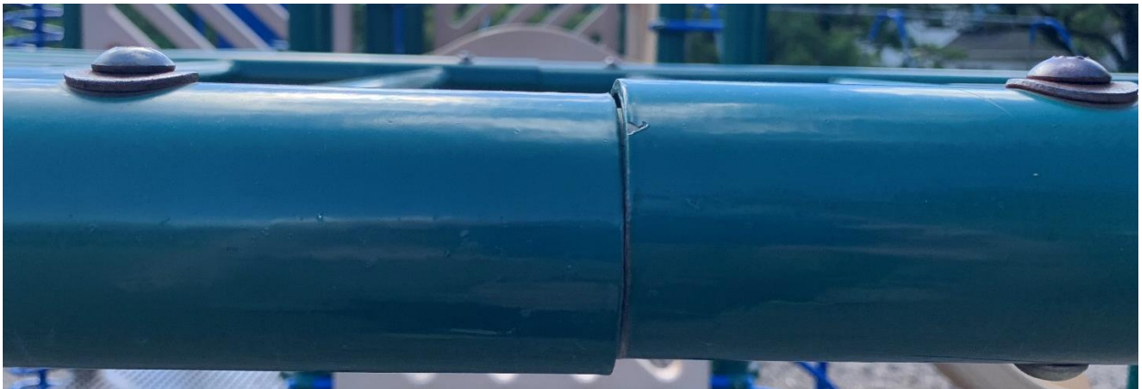
Figure 34: Section of monkey bars with minor misalignment
