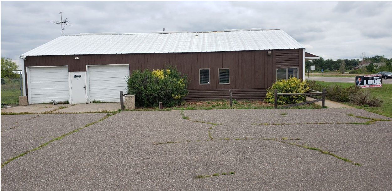
Photo 2. The side of the building and parking lot facing 147 th Avenue NW (August 15, 2022).
