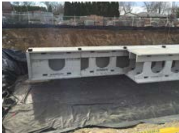
Exhibit 2: Example concrete vault storage tank (StormTrap).
