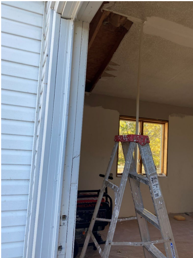
Photo 4. Work being done inside the house without building permits. October 10, 2022.
