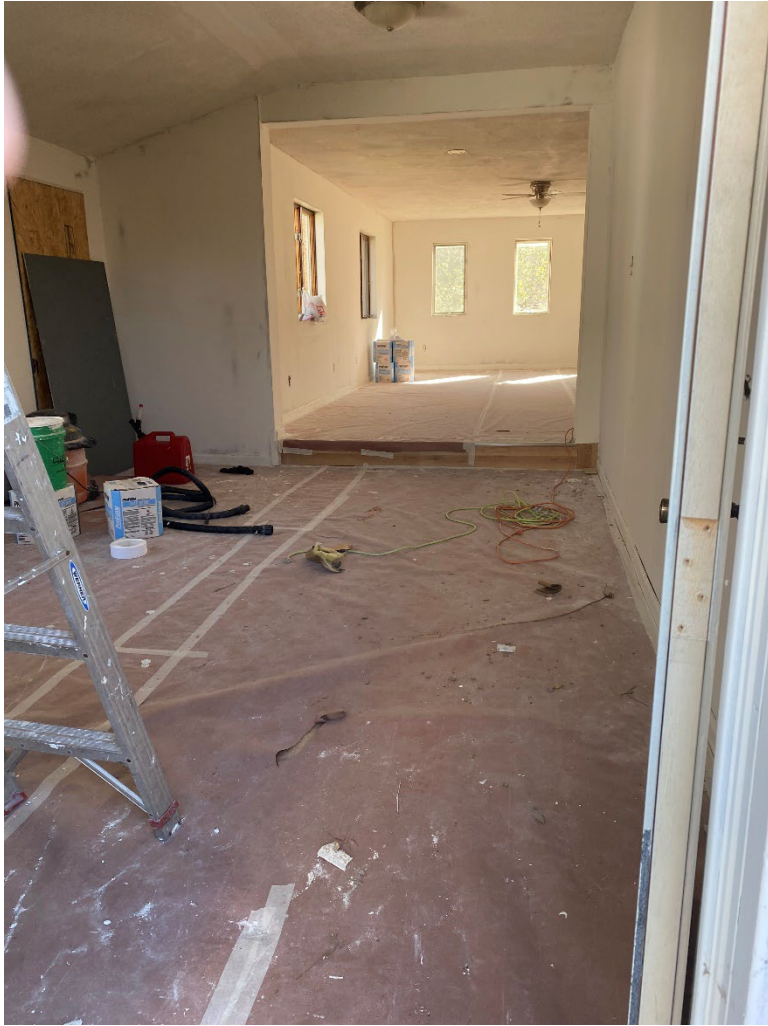
Photo 5. Work being done inside without building permits. October 10, 2022.
