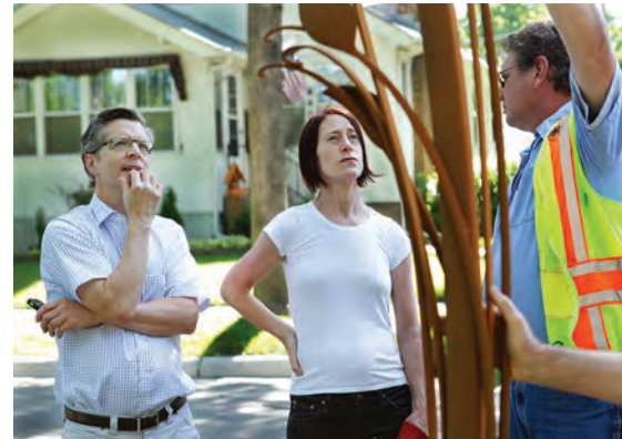
Brad Kaspari and Lisa Elias with Public Works staff installing her forged steel Flora Sign Post . Lisa Elias © 2012
