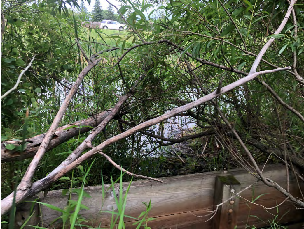
Weir between wetland 1 and Wetland 2.
