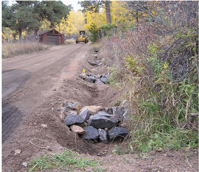
Figure 9: Rock check dams in a small ditch ( www.casfm.org/stormwater_committee/LID-Summary.htm )
