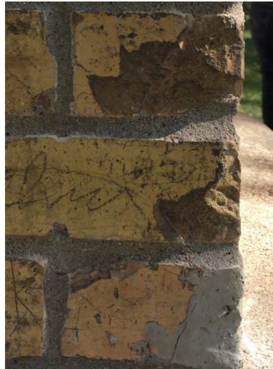
Figure 13 – Broken Brick at Corner
