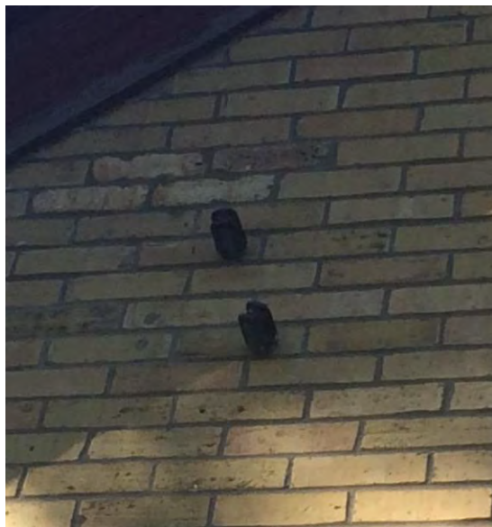
Figure 17 – Metal Brackets in Brick
