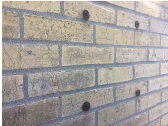
Figure 16 – Metal Brackets in Brick
