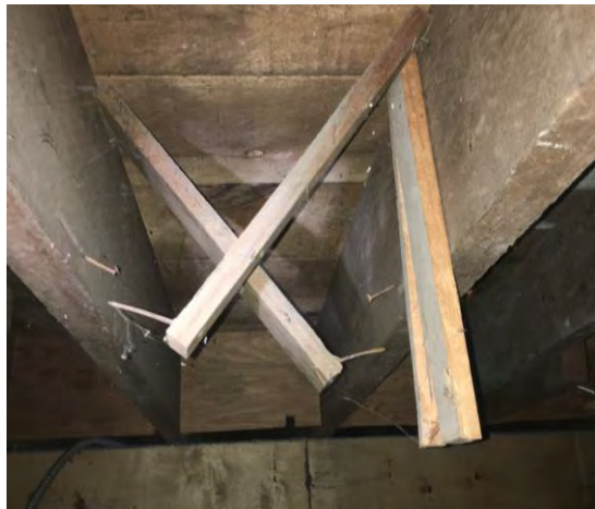
Figure 45 – Joist Cross Bracing
