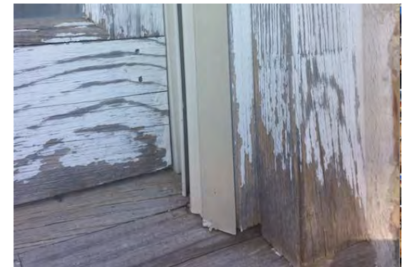
Figure 27 – Paint Chipping on Window Frame
