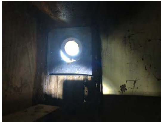
Figure 49 – Utilities Hole in Exterior Wall
