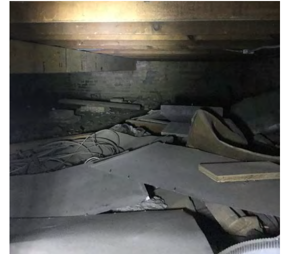
Figure 50 – Crawl Space with Debris
