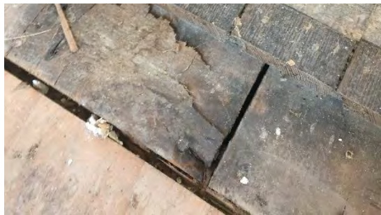
Figure 35 – Bathroom Water Damage
