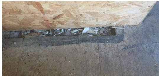
Figure 35 – Main Room, Holes in Floor
