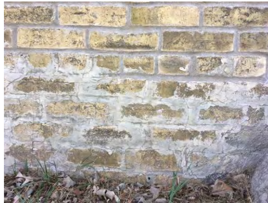
Figure 23 – Deteriorated Brick with Mortar
