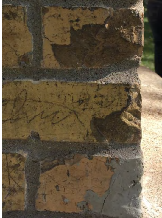
Figure 13 – Broken Brick at Corner
