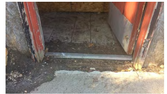
Figure 9 – Front Door Threshold
