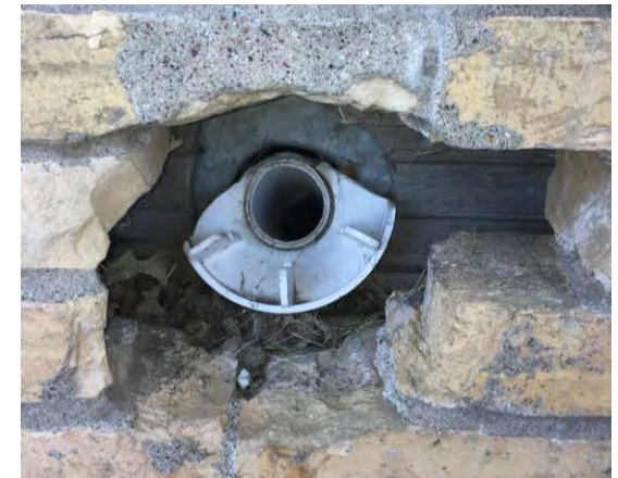
Figure 23 – Exterior Pipe Penetration
