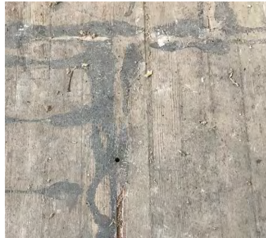
Figure 36 – Holes Along Wood Grain
