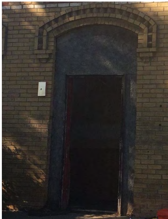
Figure 5 – Front Entrance with Particleboard
