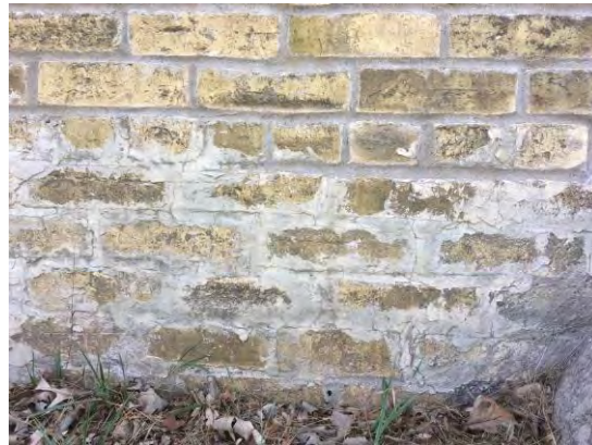
Figure 23 – Deteriorated Brick with Mortar
