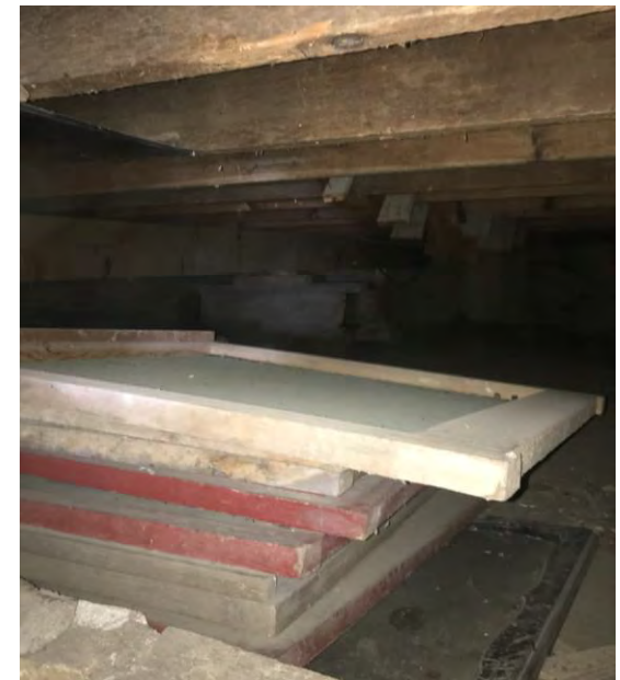
Figure 51 – Crawl Space with Debris
