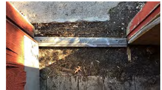
Figure 34 – Entry Hall Flooring at Threshold
