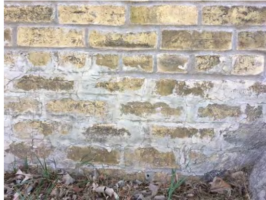
Figure 23 – Deteriorated Brick with Mortar
