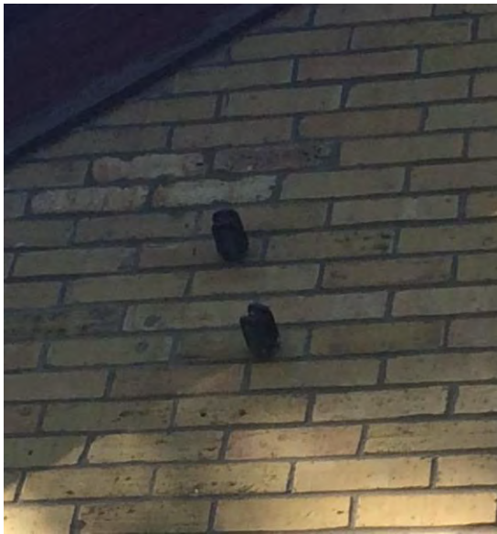
Figure 17 – Metal Brackets in Brick
