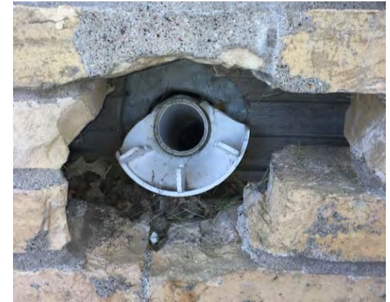
Figure 23 – Exterior Pipe Penetration
