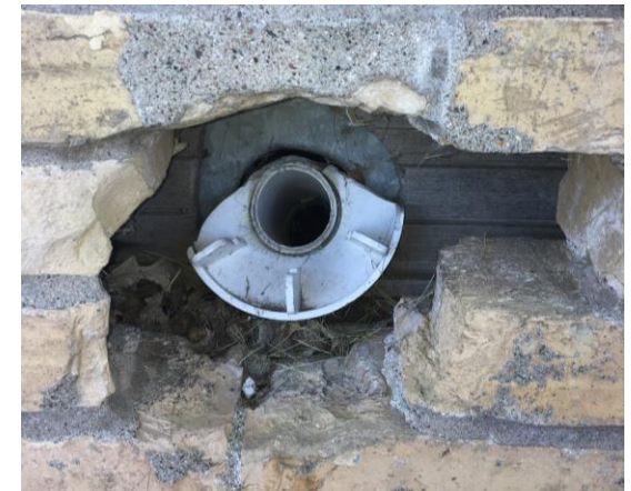
Figure 23 – Exterior Pipe Penetration
