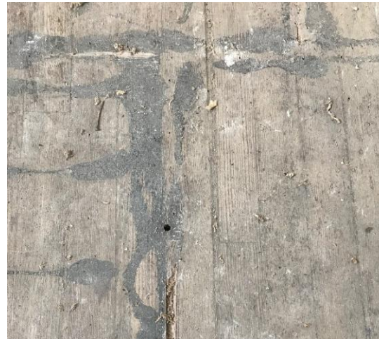
Figure 36 – Holes Along Wood Grain
