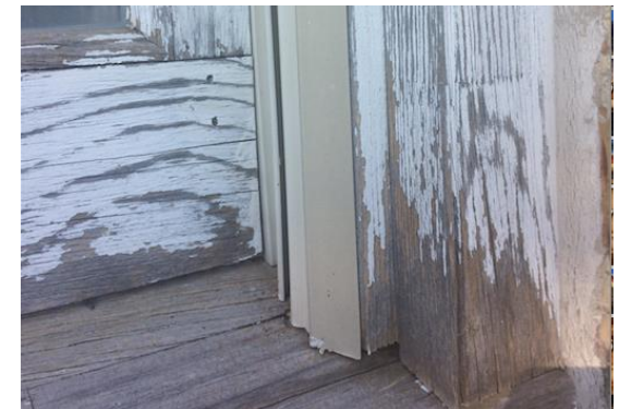
Figure 27 – Paint Chipping on Window Frame
