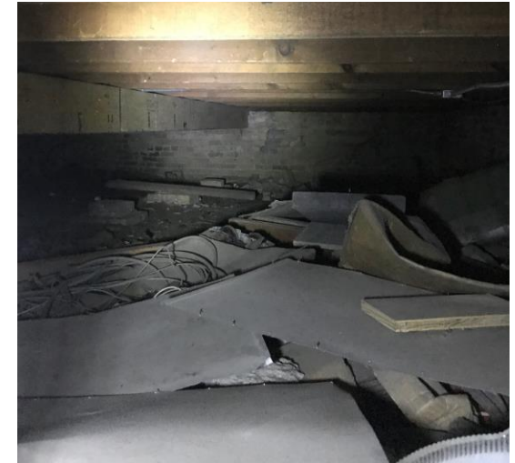
Figure 50 – Crawl Space with Debris
