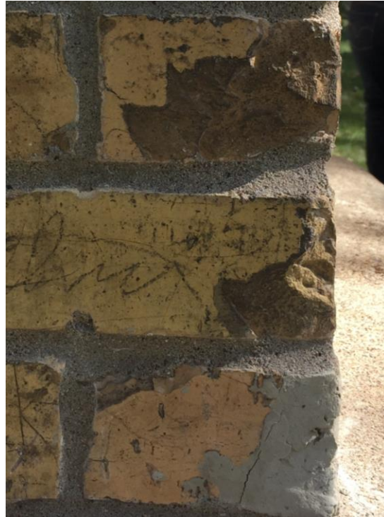
Figure 13 – Broken Brick at Corner
