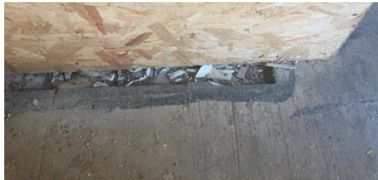
Figure 35 – Main Room, Holes in Floor
