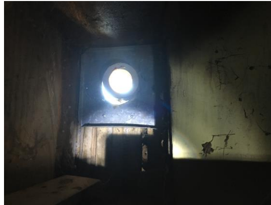
Figure 49 – Utilities Hole in Exterior Wall
