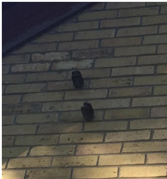
Figure 17 – Metal Brackets in Brick
