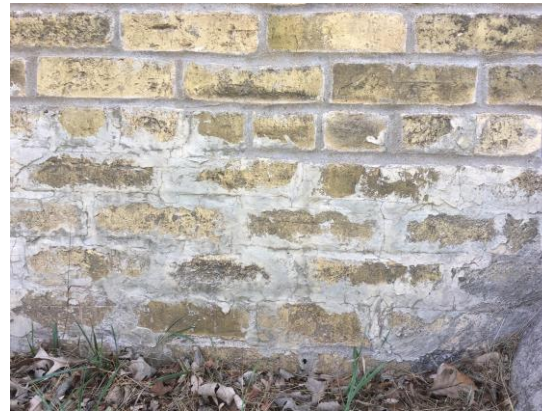
Figure 23 – Deteriorated Brick with Mortar
