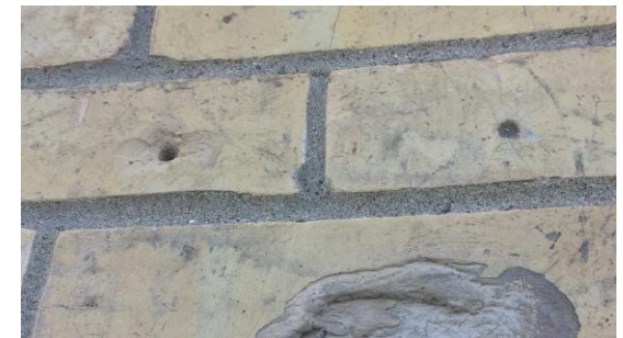
Figure 15 – Holes in Brick from Sign
