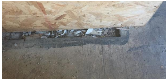
Figure 35 – Main Room, Holes in Floor
