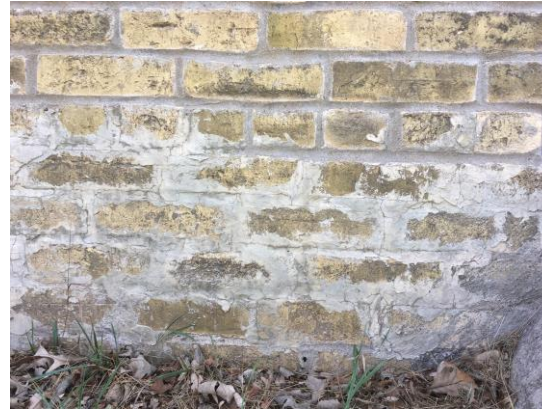
Figure 23 – Deteriorated Brick with Mortar
