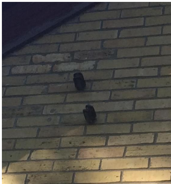
Figure 17 – Metal Brackets in Brick
