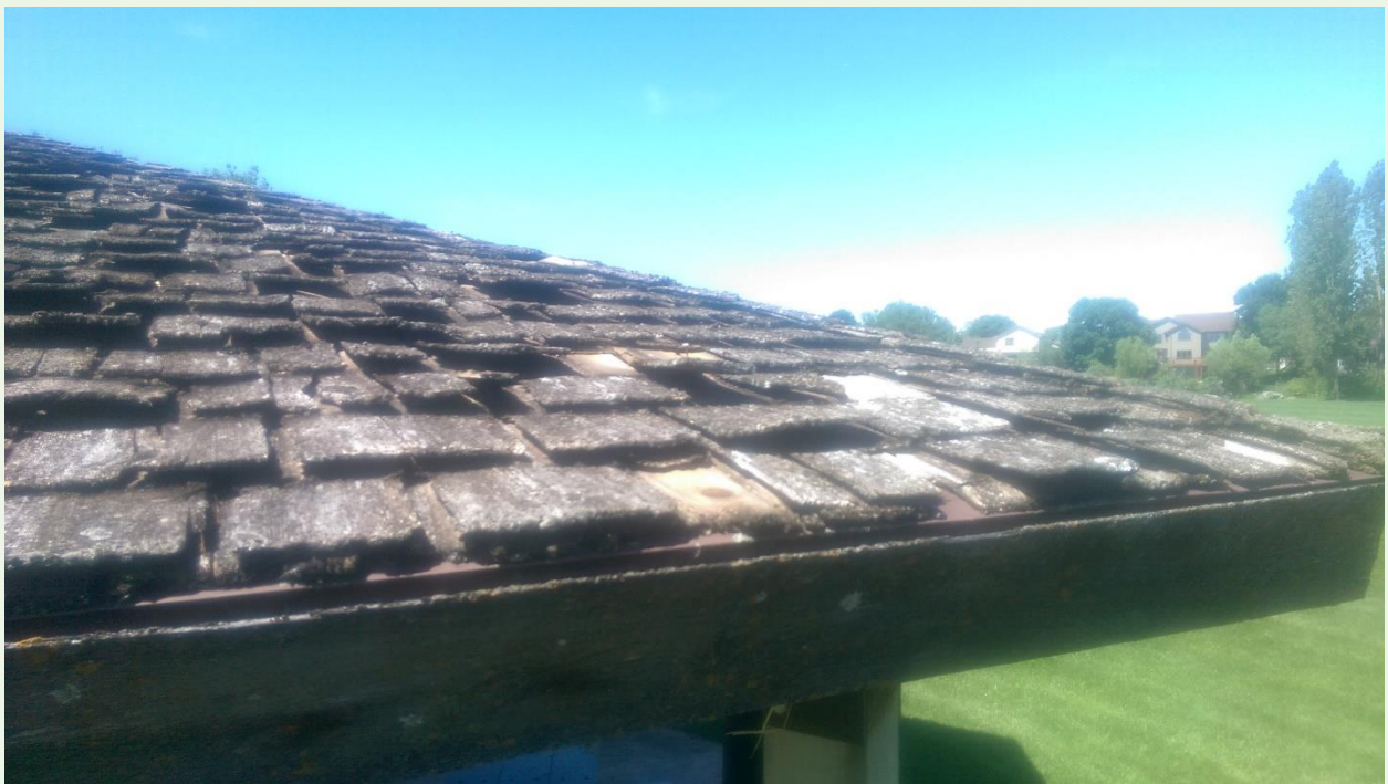
Shingle conditions (June 2018)
