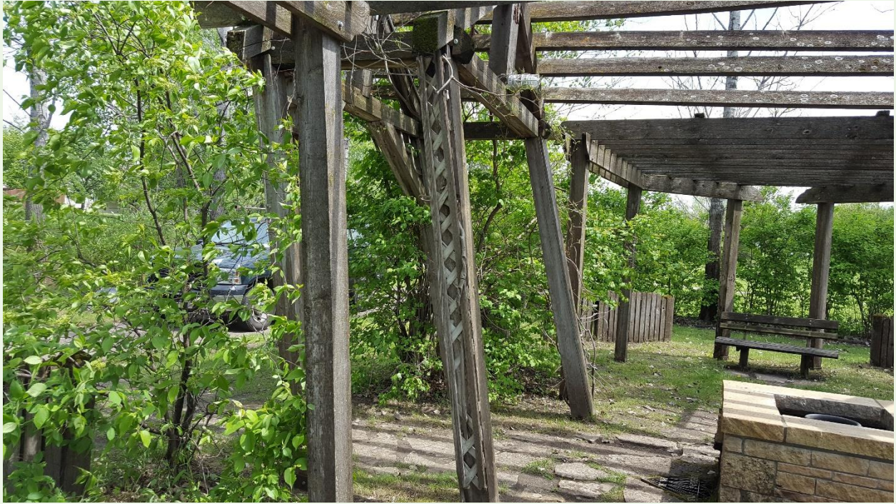
'Interior' views demonstrating column tilt from decayed base ↕
