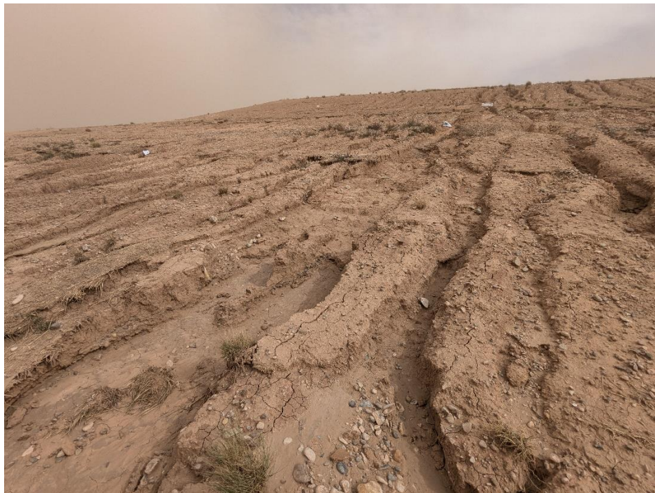
Photo 6. Erosion and Rilling along Unit 3 side slope
