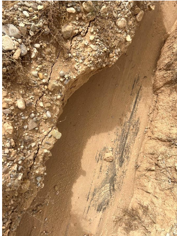
Photo 5. Geotextile exposed near base of Unit 2 side slope
