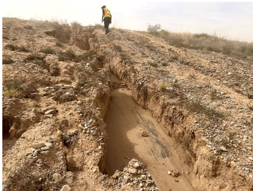
Photo 4. Erosion and Rilling with exposed geotextile along Unit 2 side slope
