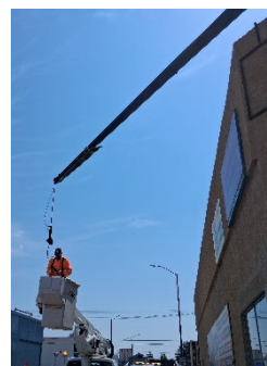
Damaged arm mast 2 nd St. & 285
