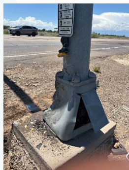
Damaged arm mast at Relief Route and S. Main St.
