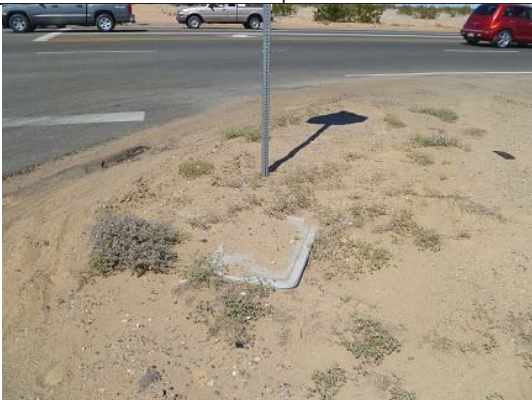
23. SEC ADOT Pull Box
