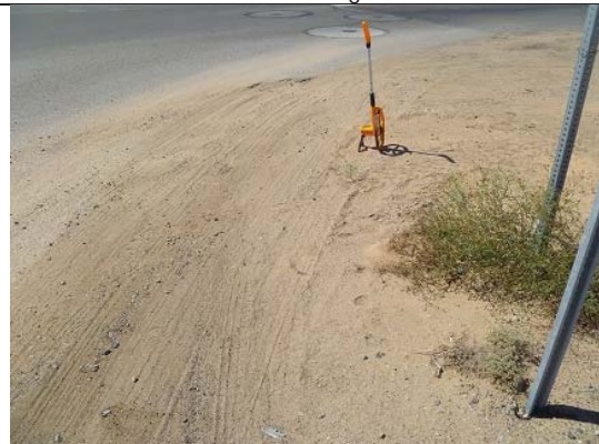
8. NEC no curb or ramps
