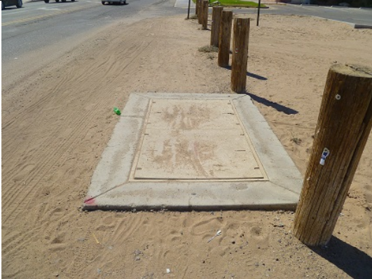
13. NWC Utility Vault by NS Access
