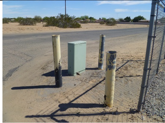
26. SWC 4 th Utility bollards
