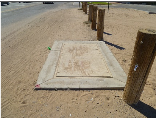
13. NWC Utility Vault by NS Access
