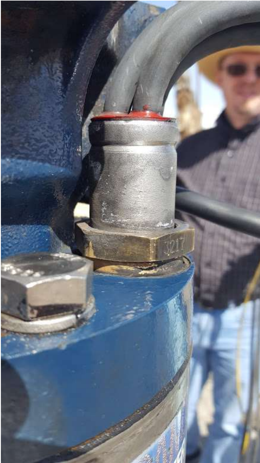
Figure 2.2.4-Electrical connector from Cable to Motor
