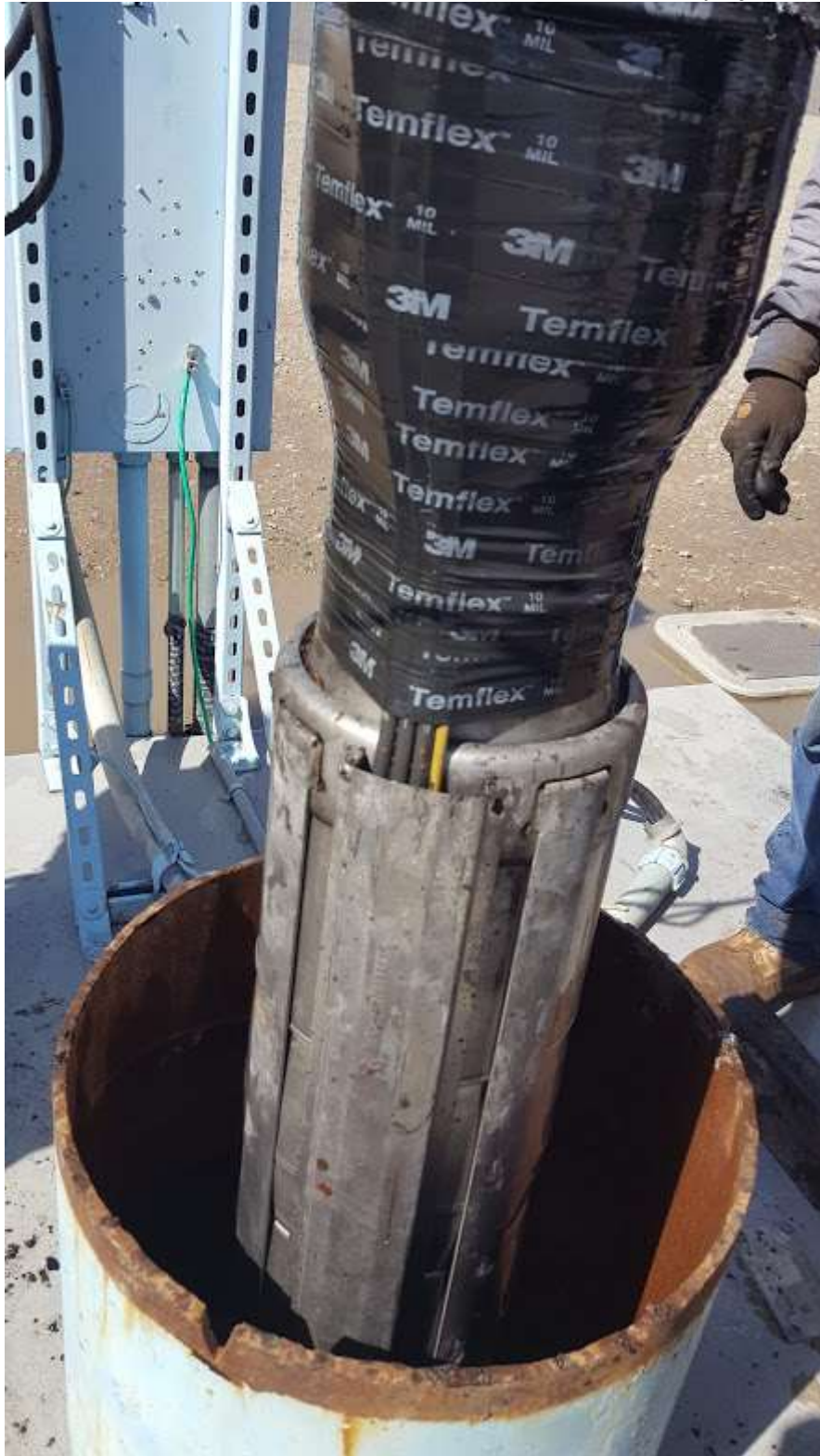
Figure 2.2.4-Pump and Motor removed, Motor hanging concentric in in well head shaft, no connection to ground
