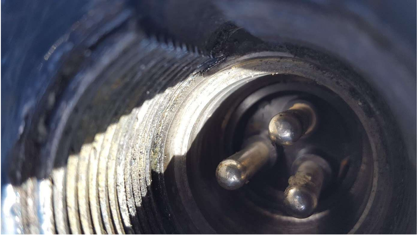
Figure 2.2.5- View of the internal components of the connector. Note: Once the cable was removed, the resistance remained low as throughout the previous measurements, pointing to internal components of the motor.
